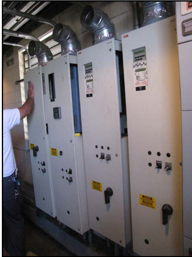
Figure 2-14. Walnut Stormwater Pumping Station: Adjustable Frequency Drives
