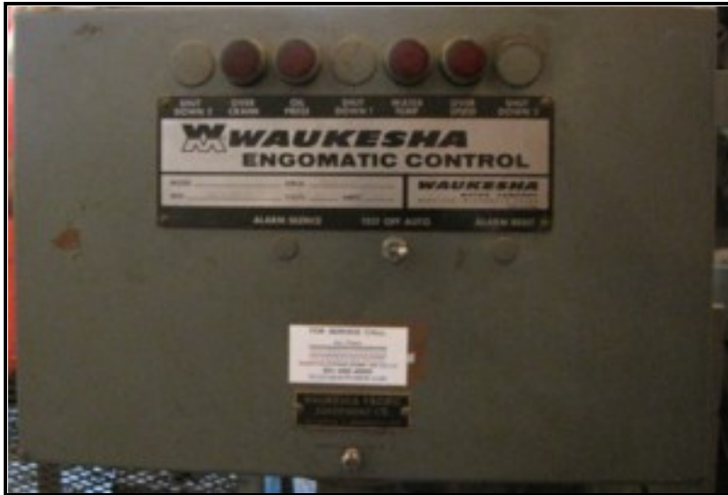
Figure 3-9. Angus Stormwater Pumping Station: Engine Control and Alarm Panel
