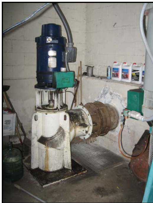
Figure 2-2. Walnut Stormwater Pumping Station: Pump 1 (30 hp).
