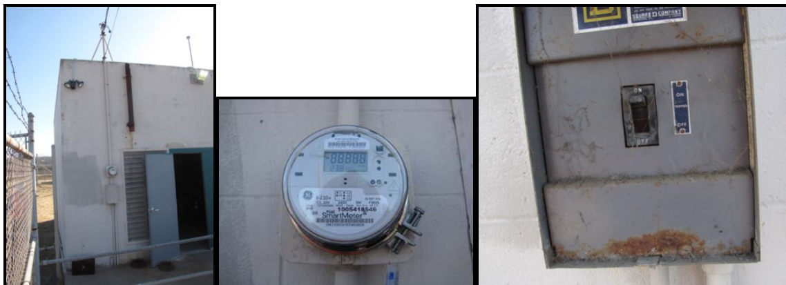
Figure 3-6. Angus Stormwater Pumping Station: Electrical Service Equipment; Overhead Service to Meter and Disconnect (left) Utility Meter (middle), and Main Service Disconnect Circuit Breaker (right)
