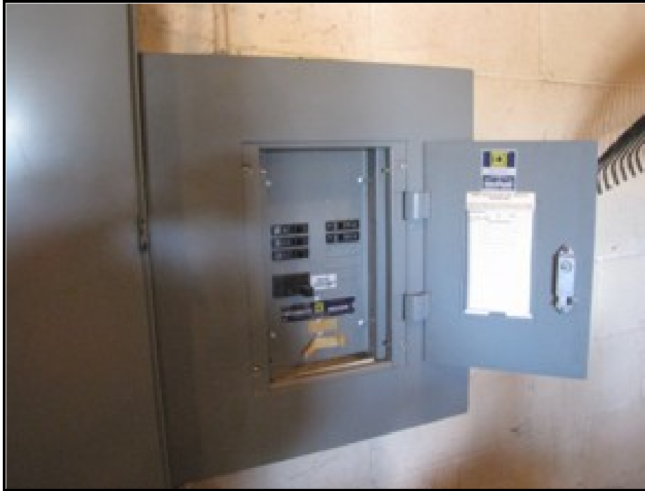
Figure 3-7. Angus Stormwater Pumping Station: Electrical Panelboard (ATS to left)
