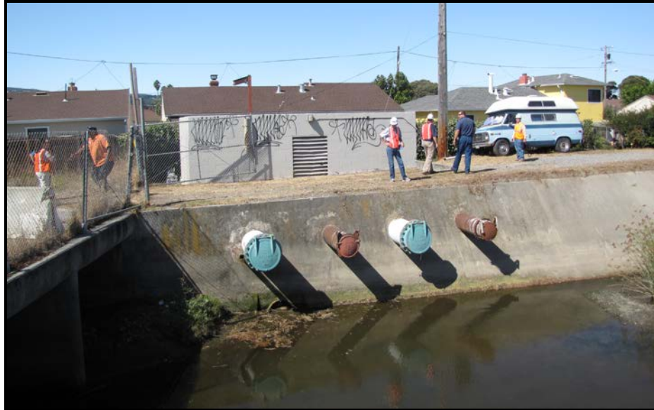
Figure 2-4. Walnut Stormwater Pumping Station: 24-inch and 16-inch Discharge Pipes
