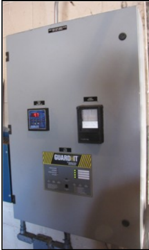
Figure 3-8. Angus Stormwater Pumping Station: Lift Station Control Panel
