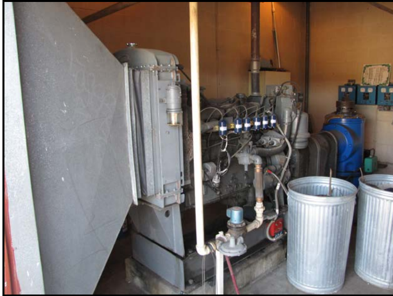
Figure 3-1. Angus Stormwater Pumping Station: Pump 1 (110 hp.)
