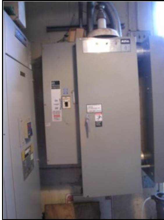
Figure 2-11. Walnut Stormwater Pumping Station: MCC (extreme left) Main Breaker, ATS (center), and Generator Breaker (extreme right, partial).
