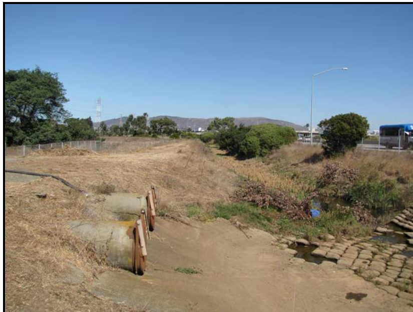
Figure 3-2. Angus Stormwater Pumping Station: 36-inch Discharge Piping and Flap Gates
