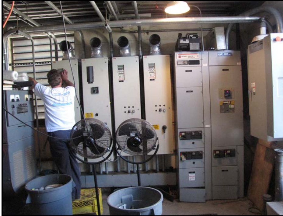
Figure 2-13. Walnut Stormwater Pumping Station: Electrical Equipment Lineup; Standby Generator (far left), AFDs (left), MCC (right) ATS and Generator Breaker (far right)
