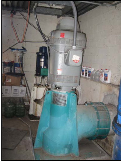
Figure 2-1. Walnut Stormwater Pumping Station: Pump 2 (75 hp).
