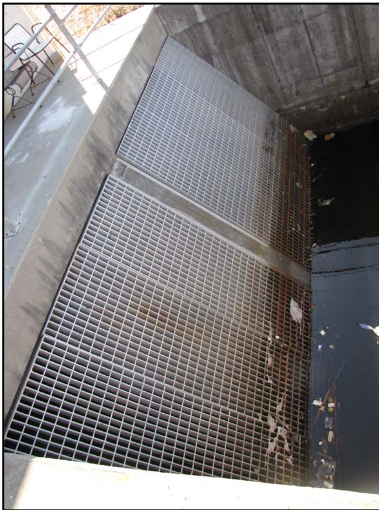
Figure 3-5. Angus Stormwater Pumping Station: Screen Grating
