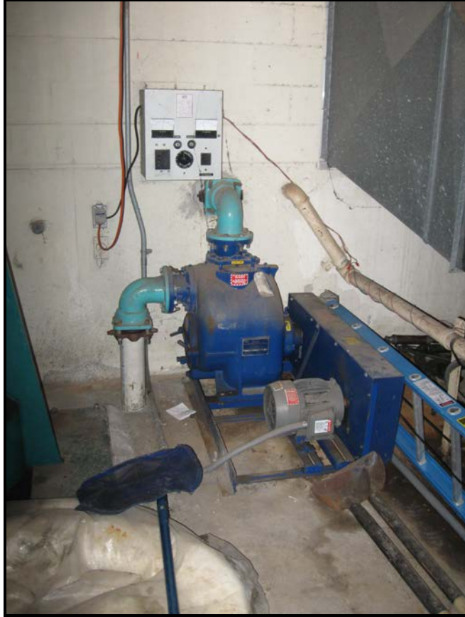
Figure 2-3. Walnut Stormwater Pumping Station: Wet Well Dewatering Pump.
