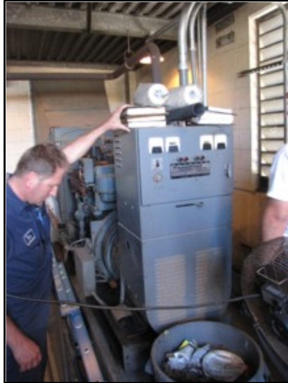
Figure 2-12. Walnut Stormwater Pumping Station: Standby Generator
