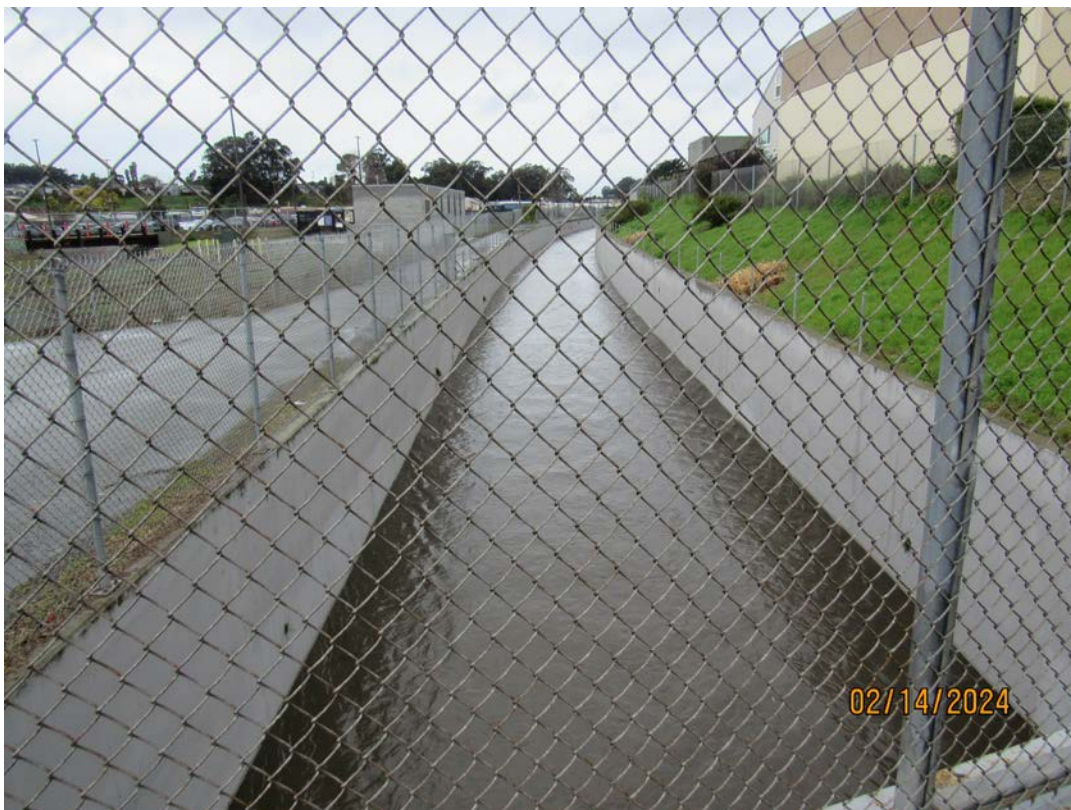
Photos 29 & 30 – Top photo shows Colma Creek looking upstream from the SSF BART Station culvert. Bottom photo shows Colma Creek looking upstream from Costco pedestrian bridge. In the bottom photo, note that walls remain graffiti free in this section. However, the channel upstream of here continues to receive fresh graffiti. Vegetation maintenance was conducted along both sides of the channel upstream of the Costco pedestrian bridge.
