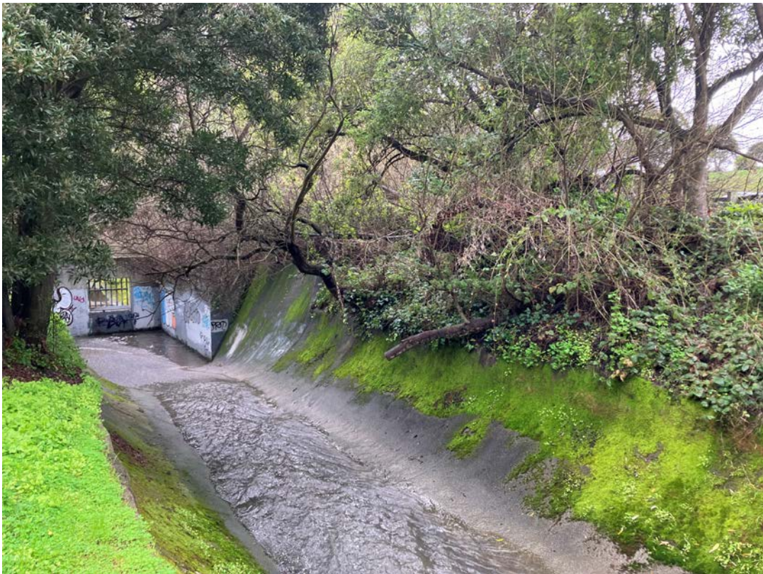
Photos 33 & 34 – Top photo shows old Colma Creek channel downstream of the El Camino Real bridge at the Mission Road intersection. Bottom photo shows Colma Creek channel facing downstream looking at the diversion structure and junction with the Old Channel.
