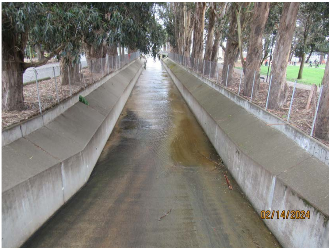
Photos 23 & 24 – Top photo shows Colma Creek looking upstream from Orange Park pedestrian bridge. Bottom photo shows Colma Creek looking downstream from Orange Park pedestrian bridge
