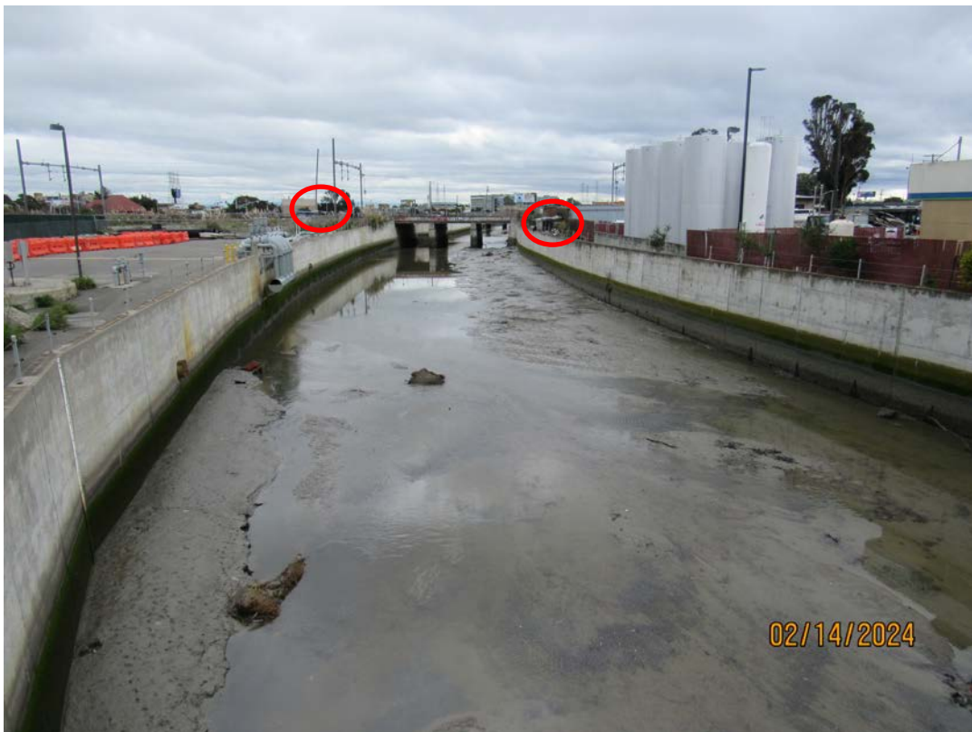
Photos 15 & 16 – Top photo shows Colma Creek looking upstream from Linden Avenue bridge. Bottom photo shows Colma Creek looking downstream from the Linden Avenue bridge. Two active encampments exist outside the channel walls in private property. OneShoreline is coordinating with SSF and other non-profit groups to address these encampments.
