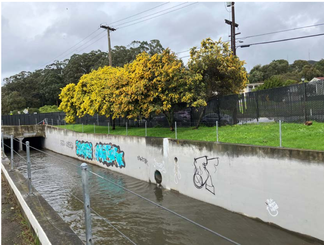
Photos 31 & 32 – Top photo shows Colma creek looking downstream Mission Road Box Culvert. Channel is free of tree limbs from the flow line. Bottom photo shows Colma Creek looking upstream at the Mission Road Box Culvert and graffiti. County recommends OneShoreline to coordinate with Colma staff to address uprooted tree leaning on the fence towards Mission Road.
