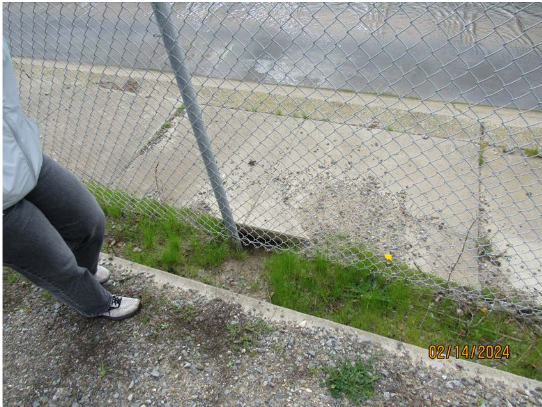
Photos 19 & 20 – Top photo shows debris accumulated at the dissipater teeth upstream of the Spruce Avenue bridge. Minor tree debris was observed caught in the teeth due to the recent rain and high wind events. County recommends OneShoreline to coordinate with SSF staff to remove the debris per the MOA between OneShoreline and SSF. Bottom photo shows void developing underneath the north sidewalk upstream of the Spruce Avenue bridge. Consultant firm has assessed the conditions of the concrete channel and recommends a geotechnical investigation be conducted to identify causes for the soil settlement. County will monitor the void in future inspections.
