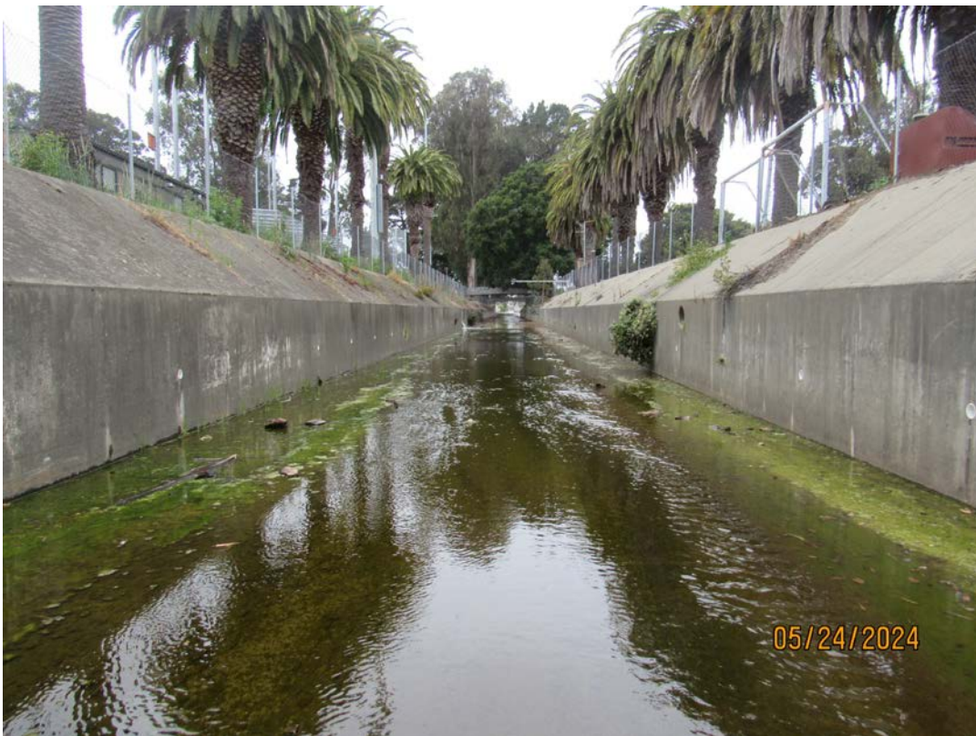
Photos 23 & 24 – Top photo shows Colma Creek looking downstream from the Orange Avenue bridge. Bottom photo shows Colma Creek looking upstream from Orange Avenue bridge. The County on behalf of OneShoreline, will be removing and trimming vegetation in the flow line in this section of channel during this year's maintenance activity.
