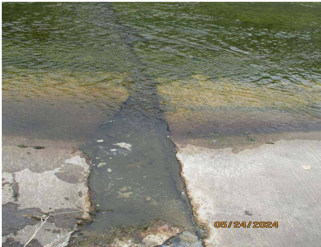
Photos 29 & 30 – Top photo shows vegetation overgrown over two culvert outfalls near BART. Vegetation clearing in this section of channel is included in this year's maintenance activities. Bottom photo shows degraded channel floor downstream from the BART box culvert. Consultant firm has assessed the conditions of the concrete channel and recommends continued monitoring of the defect in future inspections.
