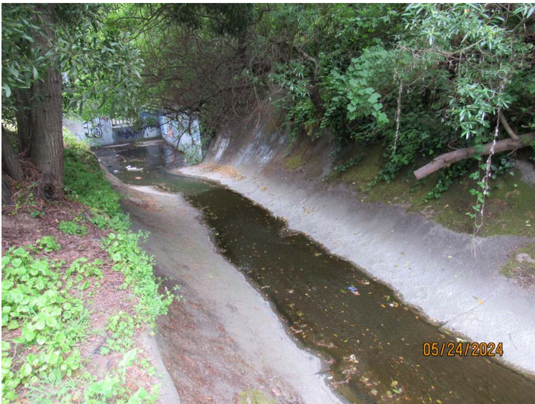
Photos 37 & 38 – Top photo shows old Colma Creek channel downstream of the El Camino Real bridge at the Mission Road intersection. Bottom photo shows Colma Creek channel facing downstream looking at the diversion structure and junction with the Old Channel.
