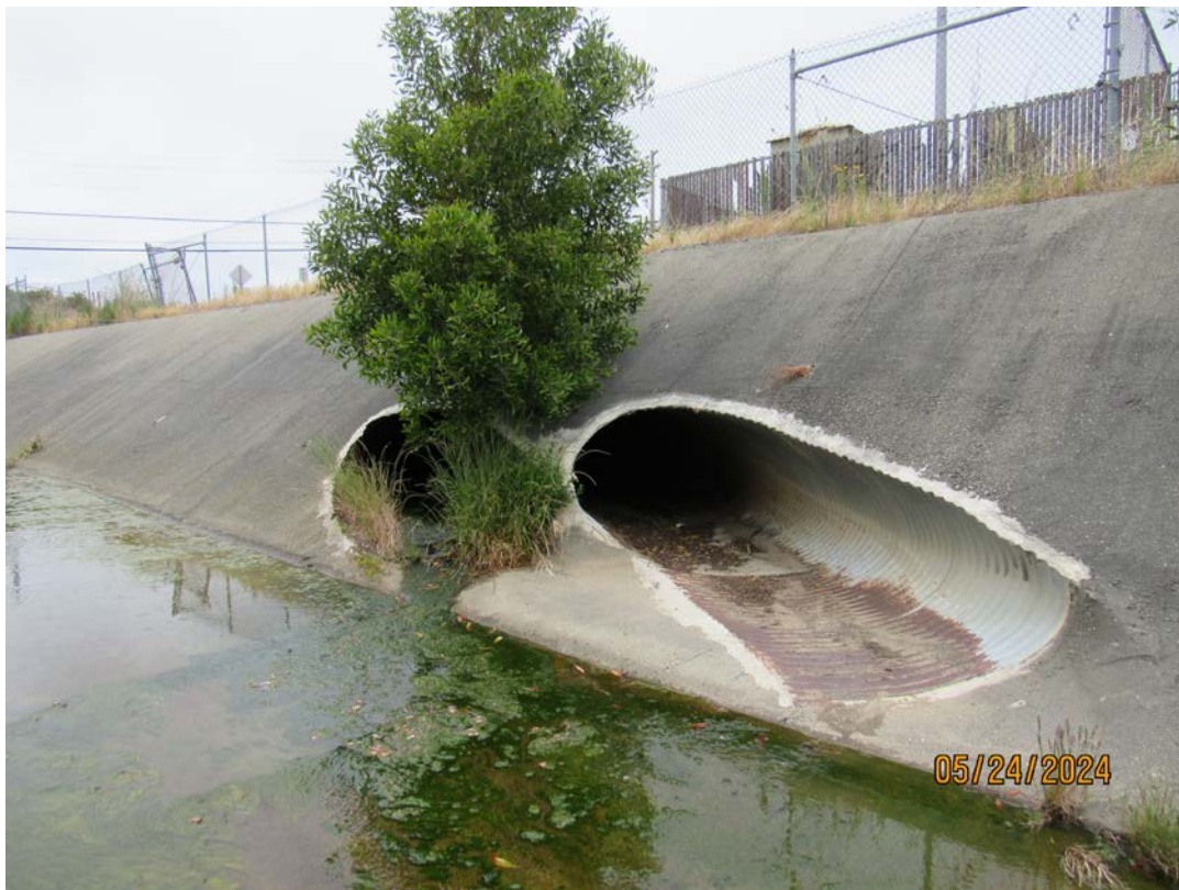
Photos 25 & 26 – Top photo shows Colma Creek looking upstream towards the 12-Mile Creek confluence. Overgrown vegetation observed in the wall joints and weepholes between the Orange Avenue bridge and 12-Mile Creek confluence. Bottom photo shows vegetation growing through a CMP culvert outlet downstream of the Centennial Way pedestrian bridge. Vegetation clearing in this section of channel is included in this year's maintenance activities.
