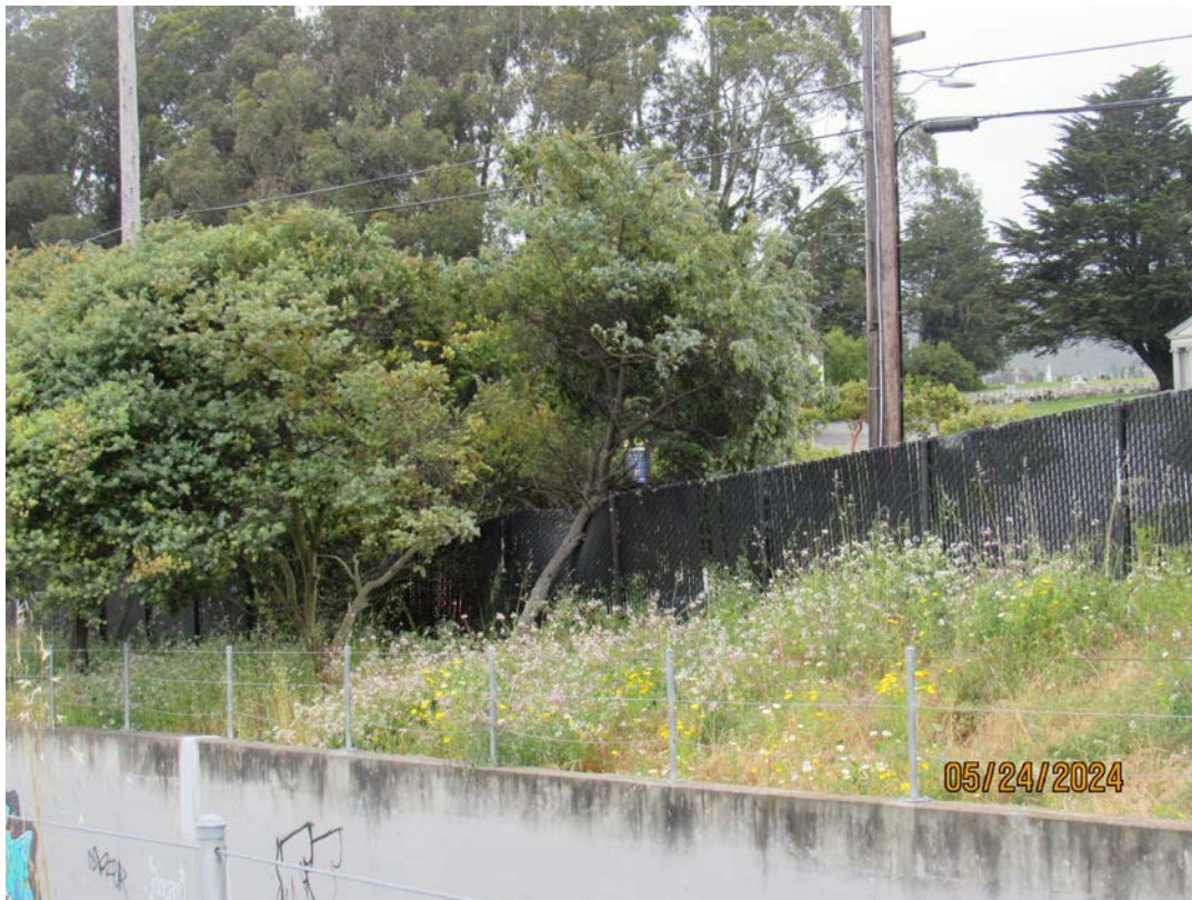
Photos 35 & 36 – Top photo shows Colma creek looking downstream from the outlet of Mission Road Box Culvert. Channel is free of tree limbs from the flow line. Bottom photo shows split tree limb falling on fence near the Mission Road Box Culvert. County recommends OneShoreline to coordinate with Colma staff to address uprooted tree leaning on the fence towards Mission Road.
