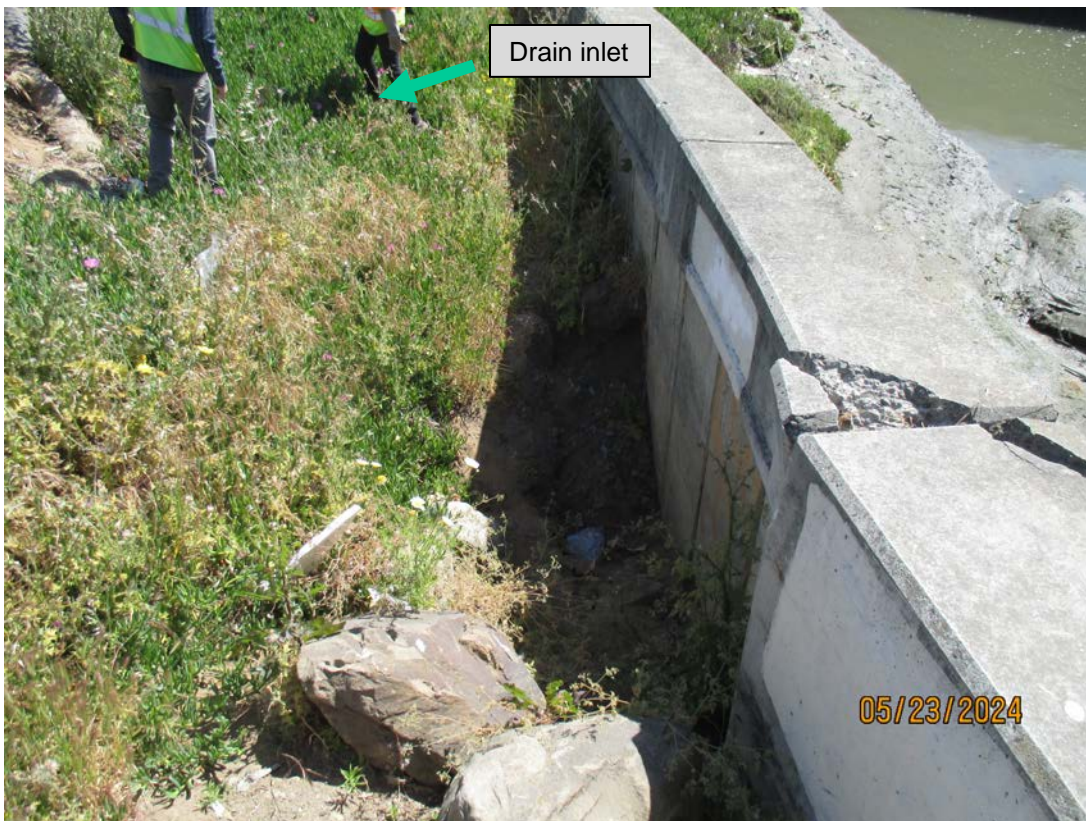
Photos 13 & 14 – Top photo shows damage on channel wall and partially blocked culvert outfall downstream from the Produce Avenue bridge facing the Hwy 101 crossing. Bottom photo shows void outside the channel wall. County recommends continuing to monitor the area and contacting Caltrans to clear the drain inlet.
