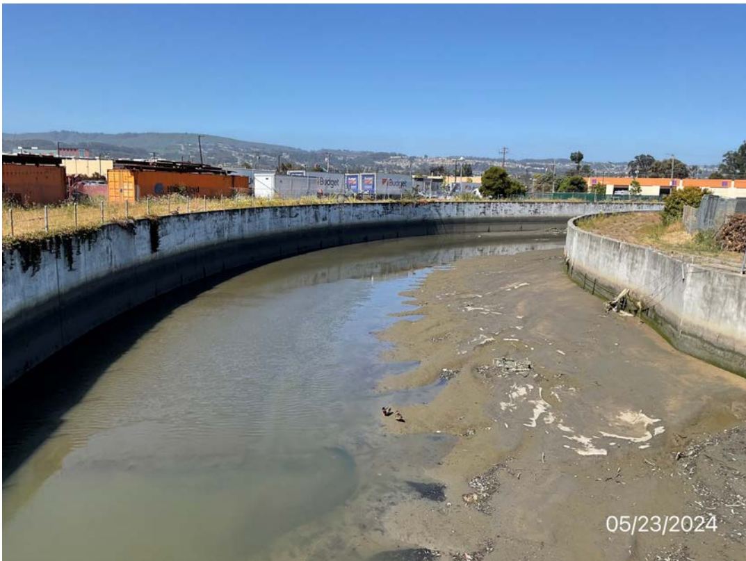
Photos 11 & 12 – Top photo shows Colma Creek looking downstream from the Produce Avenue bridge facing the Hwy 101 crossing. Bottom photo shows Colma Creek looking upstream from the Produce Avenue bridge.
