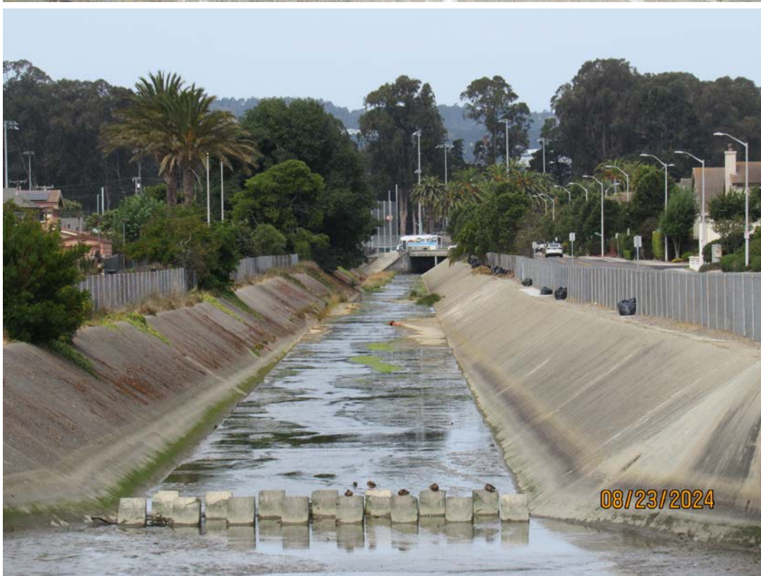
Photos 21 & 22 – Top photo shows minor debris accumulated at the dissipator teeth upstream of the Spruce Avenue bridge. Bottom photo shows channel upstream of dissipator teeth where vegetation clearing conducted by the County on behalf of OneShoreline, has been completed on the left side of the channel and is still ongoing along the right side. 11
