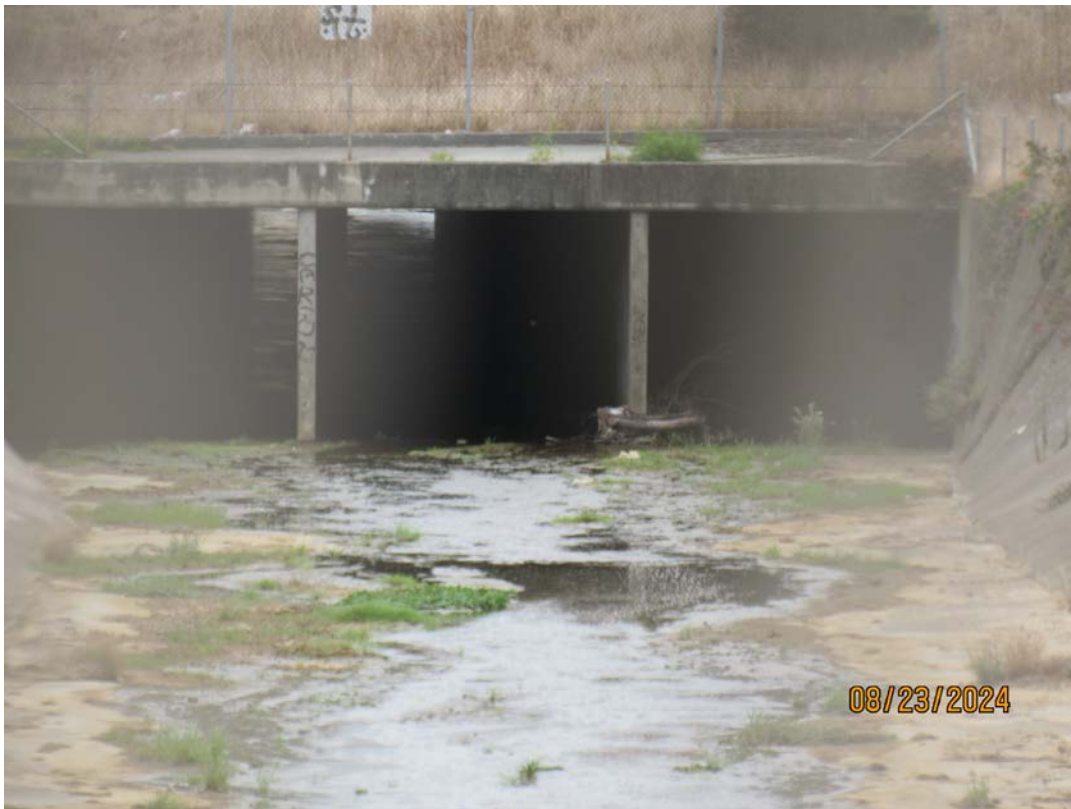
Photos 31 & 32 – Top photo shows Colma Creek looking downstream from the SSF BART Station culvert. Bottom photo shows Colma Creek looking downstream from the pedestrian trail near Costco at the box culvert.
