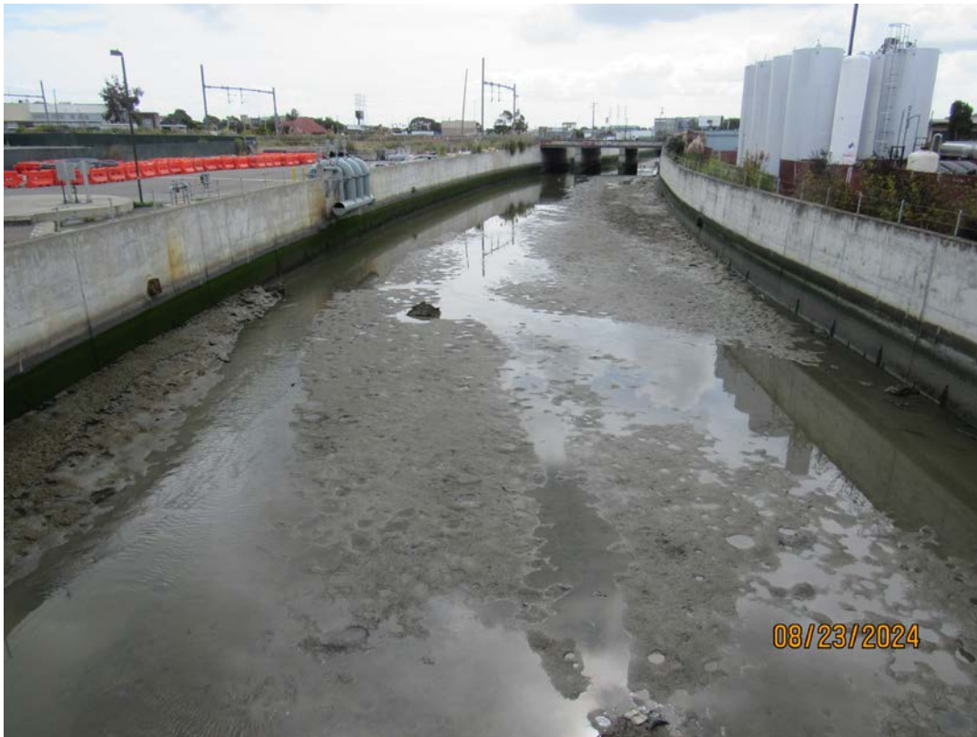
Photos 17 & 18 – Top photo shows Colma Creek looking upstream from Linden Avenue bridge. Bottom photo shows Colma Creek looking downstream from the Linden Avenue bridge. The areas outside the channel walls were clear of active encampments.
