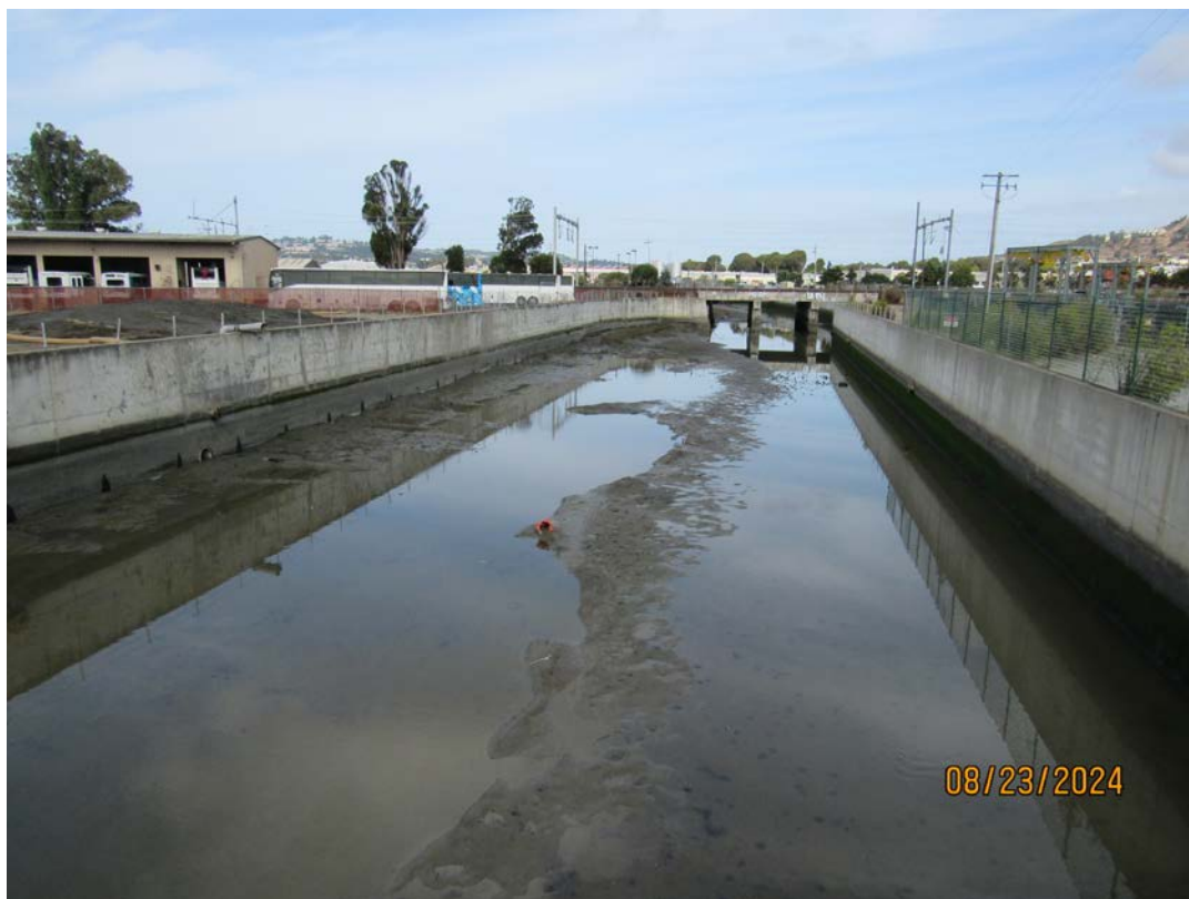
Photos 15 & 16 – Top photo shows Colma Creek looking downstream from the San Mateo Avenue bridge. Access roads in top photo were cleared of vegetation and debris as part of this year's maintenance work. Bottom photo shows Colma Creek looking upstream from the San Mateo Avenue bridge. This section was dredged of sediment by the County contractor on behalf of OneShoreline as part of this year's maintenance work.
