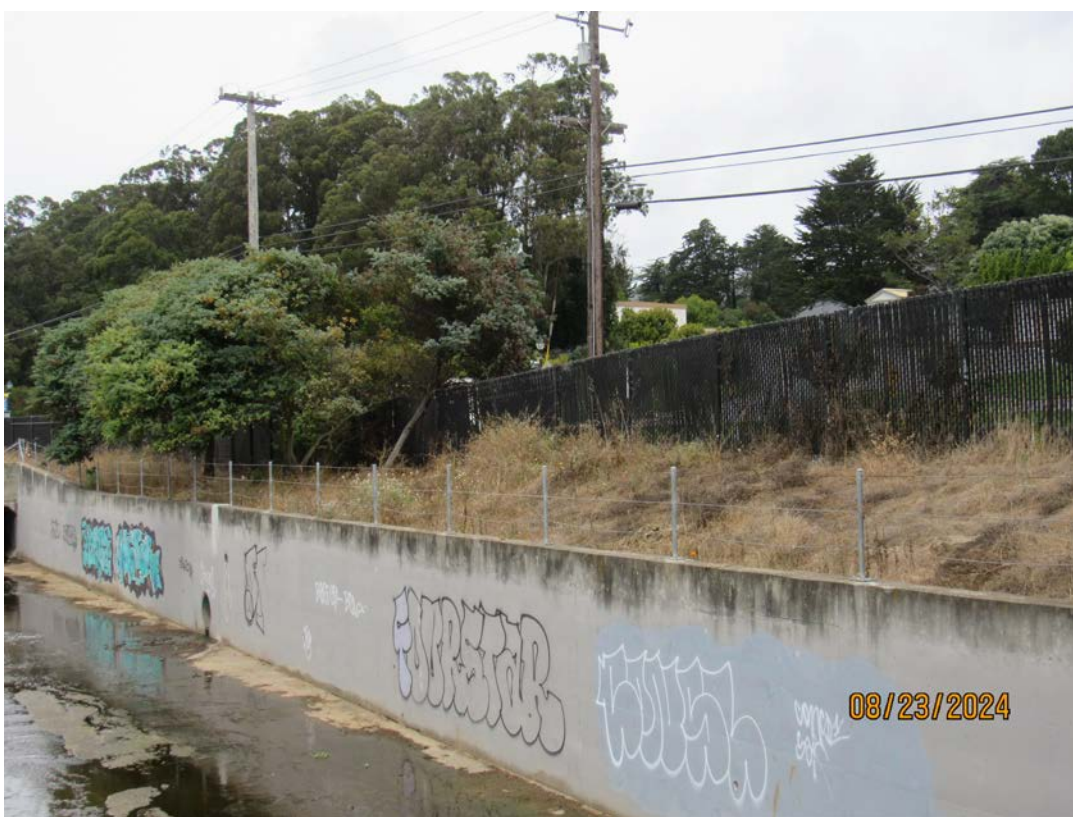
Photos 35 & 36 – Top photo shows Colma creek looking downstream from the outlet of Mission Road Box Culvert. Bottom photo shows split tree limb falling on fence near the Mission Road Box Culvert. County recommends OneShoreline to coordinate with Colma staff to address uprooted tree leaning on the fence towards Mission Road.
