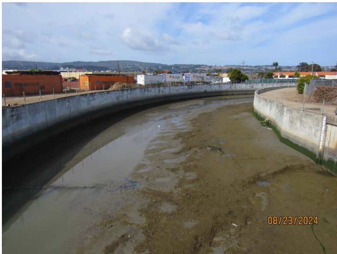
Photos 11 & 12 – Top photo shows Colma Creek looking downstream from the Produce Avenue bridge facing the Hwy 101 crossing. Trash and illegal dumping related to homeless encampment activities under the Produce Ave bridge were visible. Bottom photo shows Colma Creek looking upstream from the Produce Avenue bridge. Access roads in bottom photo were cleared of vegetation and debris by the County on behalf of OneShoreline as part of this year's maintenance work
