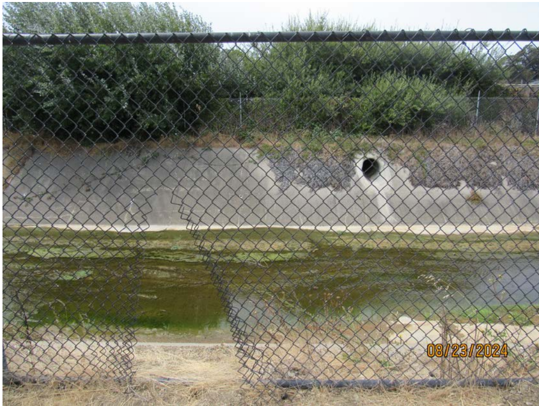
Photos 29 & 30 – Top photo shows area near Antoinette where illegal skate park and debris was removed as part of this year's maintenance activities by the County contractor on behalf of OneShoreline. Bottom photo shows fence cut along the Centennial trail near the BART station. Staff from the City of SSF Parks and Recreation Department were informed and have made the repair.
