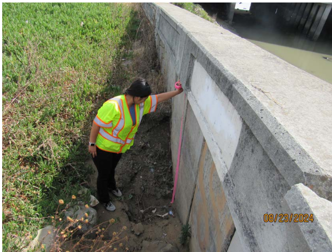
Photos 13 & 14 – Top photo shows damage on channel wall and partially blocked culvert outfall downstream from the Produce Avenue bridge facing the Hwy 101 crossing. Bottom photo shows void outside the channel wall. County recommends continuing to monitor the area and contacting Caltrans to clear the drain inlet.
