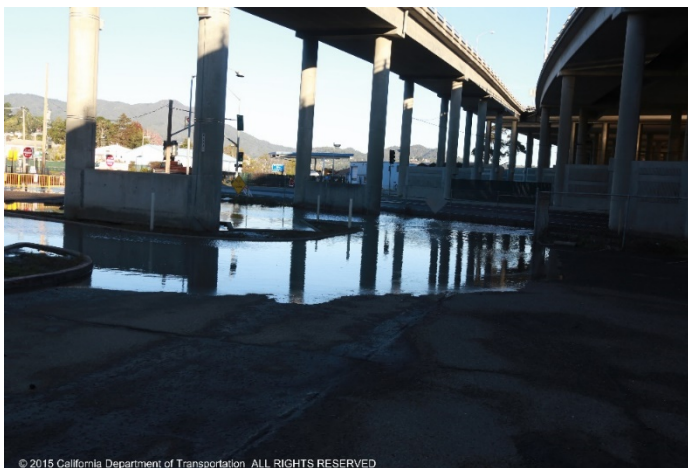
FLOODING UNDER HIGHWAY RAMPS
