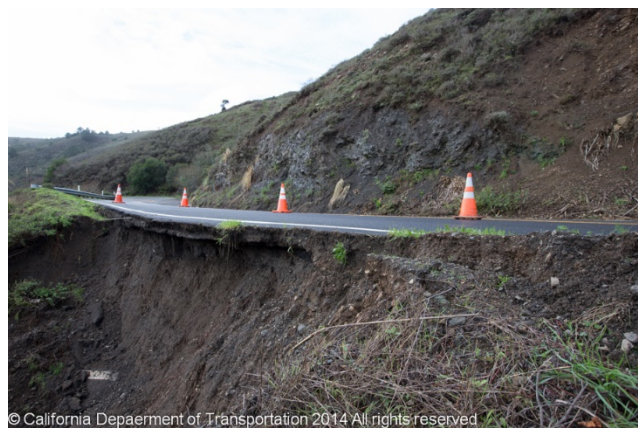
EROSION CAUSING ROADWAY HAZARD
