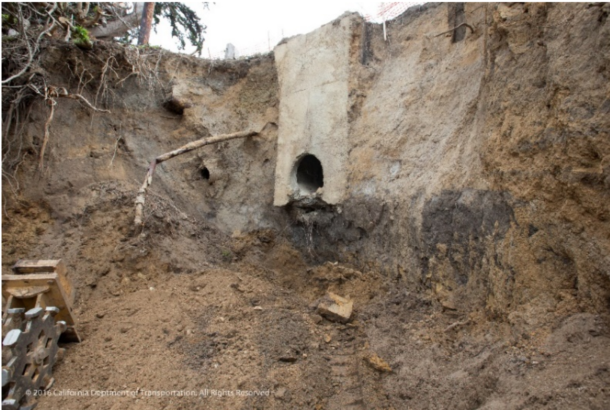
DAMAGED CULVERT UNDER REPAIR IN DISTRICT 4
