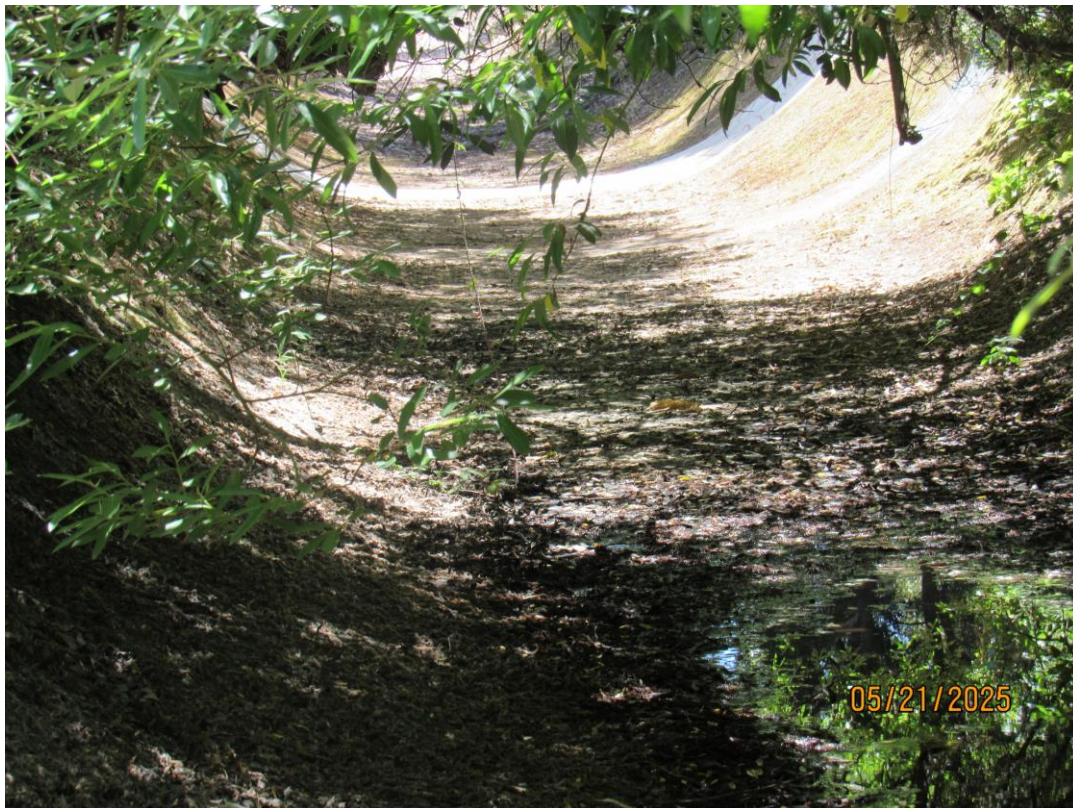
Photos 33 & 34 – Top photo shows old Colma Creek channel downstream of the El Camino Real bridge at the Mission Road intersection. Bottom photo shows Colma Creek channel facing downstream looking downstream of Old Channel.
