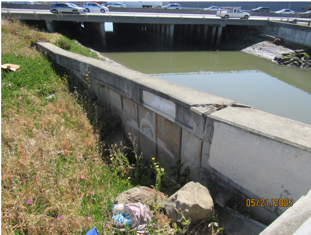
Photos 13 & 14 – Top photo shows damage on channel wall and partially blocked culvert outfall downstream from the Produce Avenue bridge facing the Hwy 101 crossing. Bottom photo shows void outside the channel wall. County recommends continuing to monitor the area and contacting Caltrans to clear vegetation at the drain inlet.
