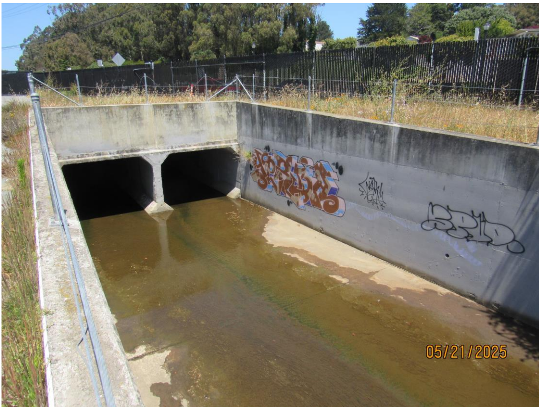
Photos 31 & 32 – Top and bottom photo shows Colma Creek looking upstream at the Mission Road Box Culvert.
