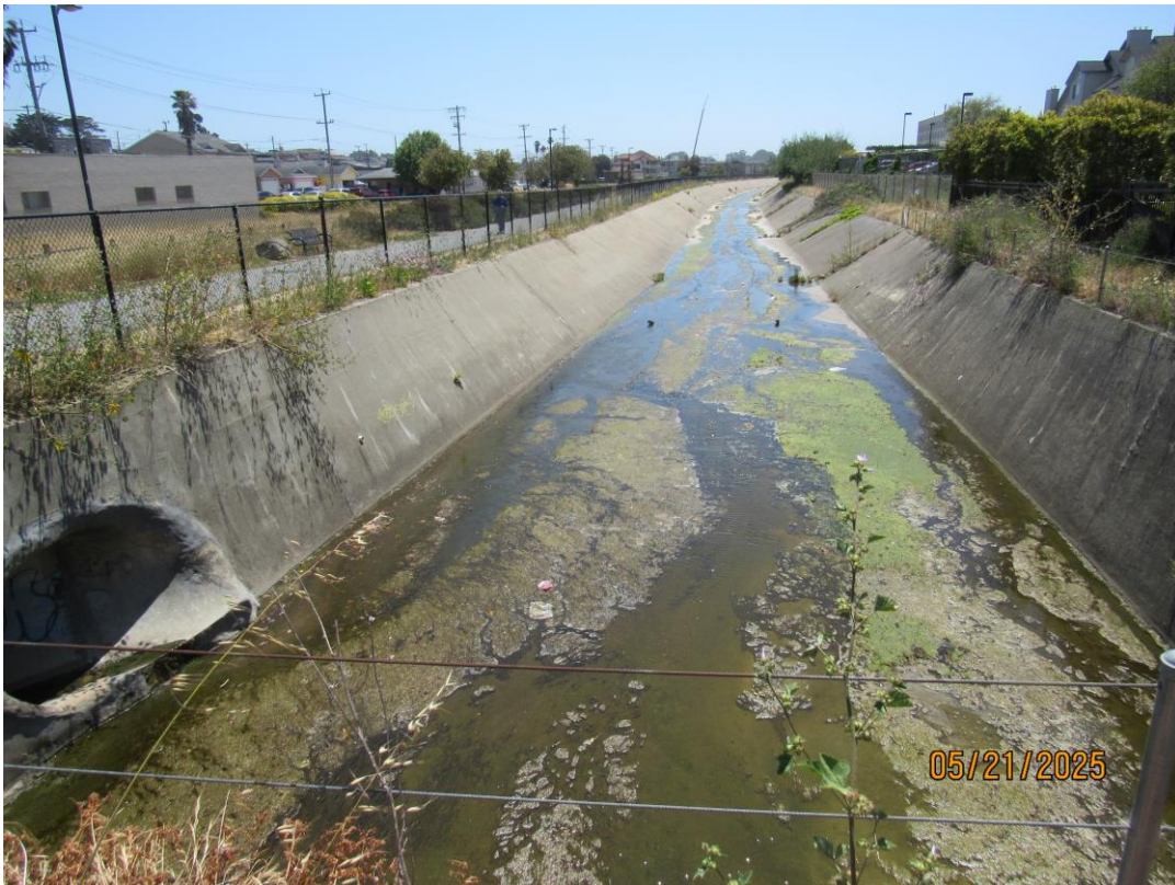
Photos 27 & 28 – Top photo shows degraded channel floor downstream from the BART box culvert. The 2023 condition assessment of the concrete channel in this section recommends continued monitoring of the defect in future inspections. Bottom photo shows culvert downstream from the SSF BART Station.
