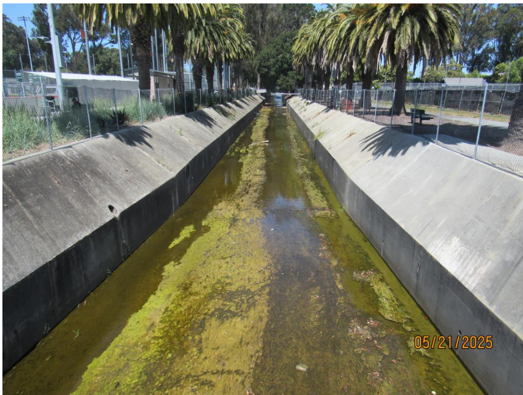
Photos 23 & 24 – Top photo shows Colma Creek looking downstream from the Orange Avenue bridge. Bottom photo shows Colma Creek looking upstream from Orange Avenue bridge.
