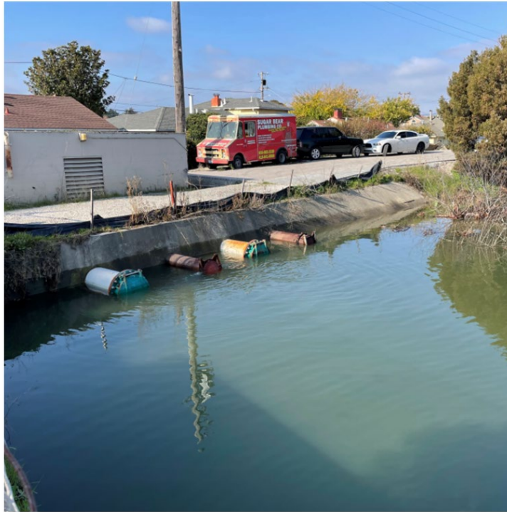
Walnut Pump Station
