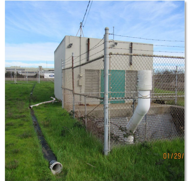
Angus Pump Station
