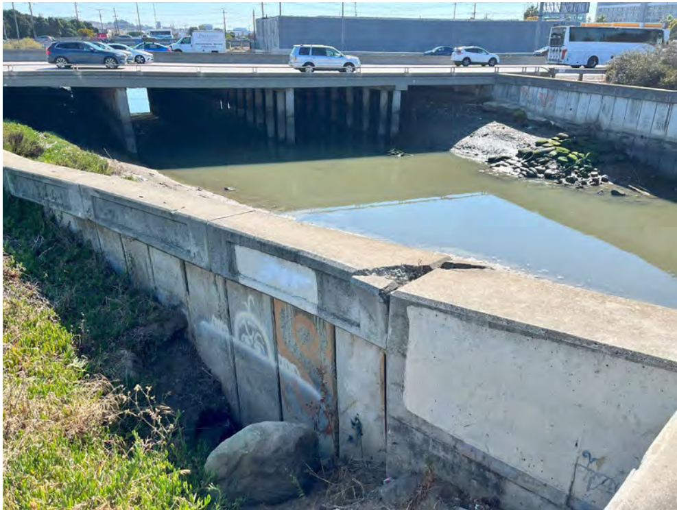
Photos 11 & 12 — Top photo shows damage on channel wall and partially blocked culvert outfall downstream from the Produce Avenue bridge facing the Highway 101 crossing. Bottom photo shows void outside the channel well. Caltrans has cleared vegetation at the drain inlet.
