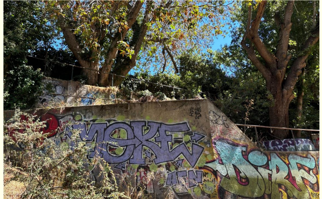
Picture of a concrete structure creating a pinch point that would be removed during channel widening
