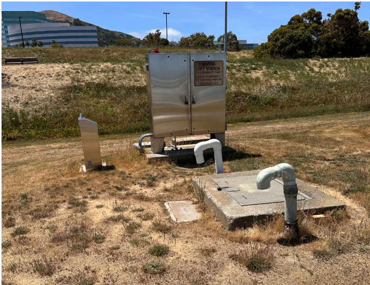
Photo 2. Harbormaster Lift Station (Lift Station #1)
