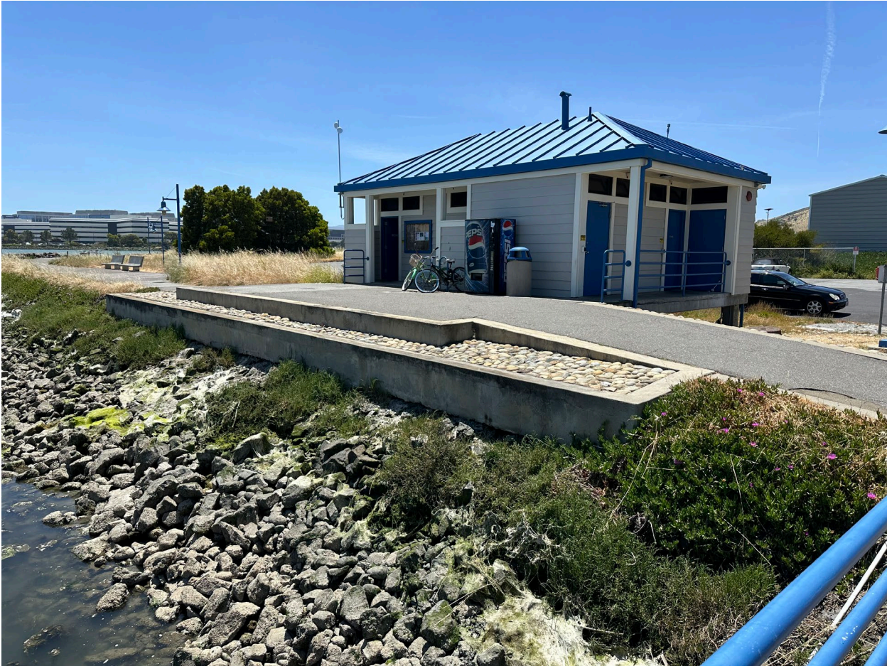
Photo 1: Bathroom on Shoreline Revetment
