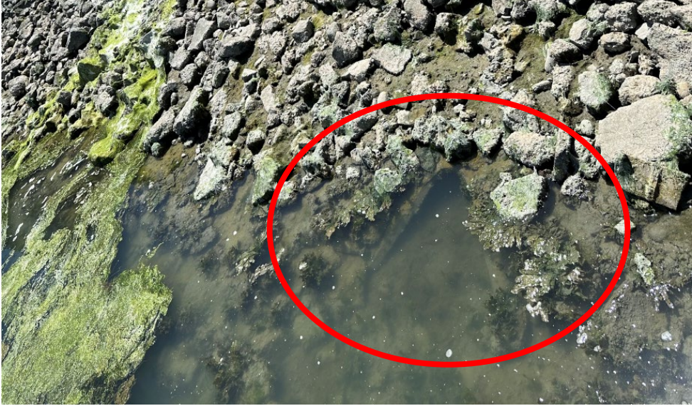
Photo 3. Submerged Outfall in the Brisbane Marina
