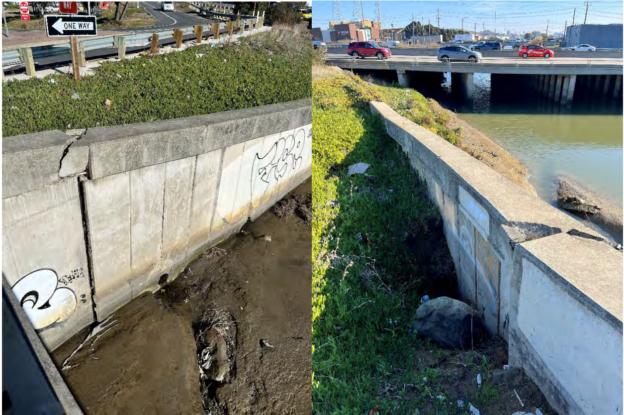
Photos 13 & 14 — Top photos show damage on channel wall and partially blocked culvert outfall downstream from the Produce Avenue bridge facing the Highway 101 crossing, and void outside the channel well.
