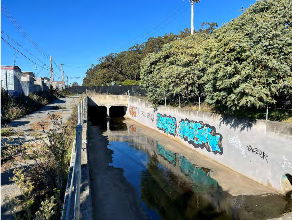
Photos 33 & 34 — Top and bottom photo shows Colma Creek looking upstream at the Mission Road Box Culvert.
