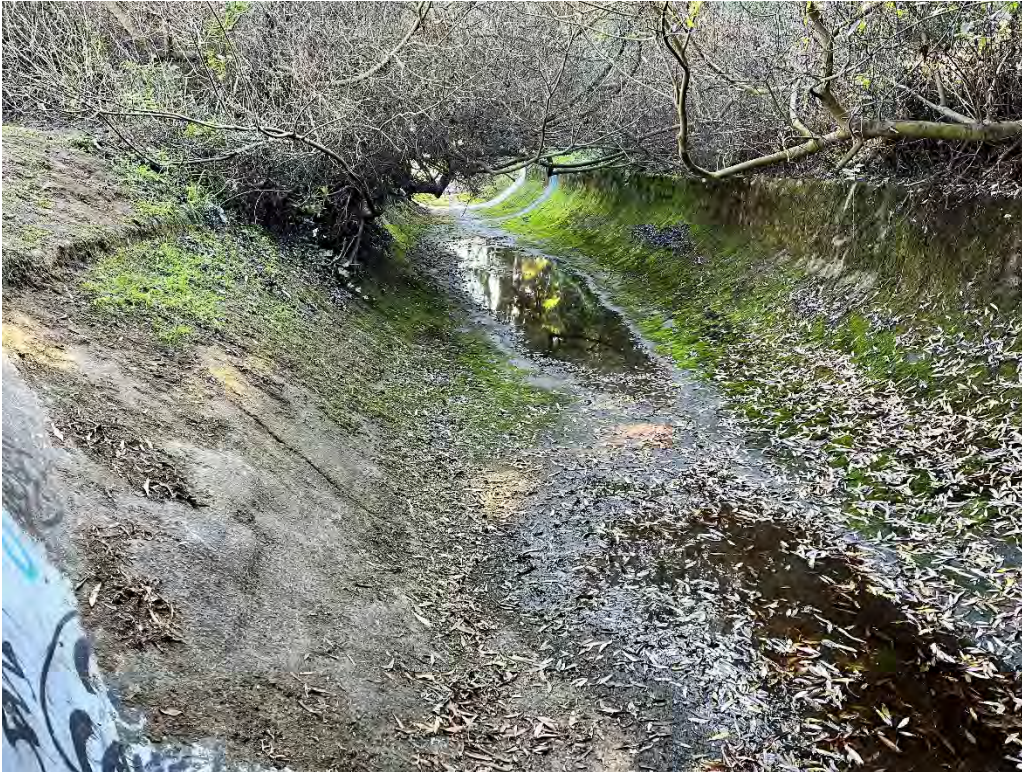
Photos 35 & 36 — Top photo shows Old Colma Creek channel downstream of the El Camino Real Bridge at the Mission Road intersection. Bottom photo shows Colma Creek channel looking downstream of Old Channel.
