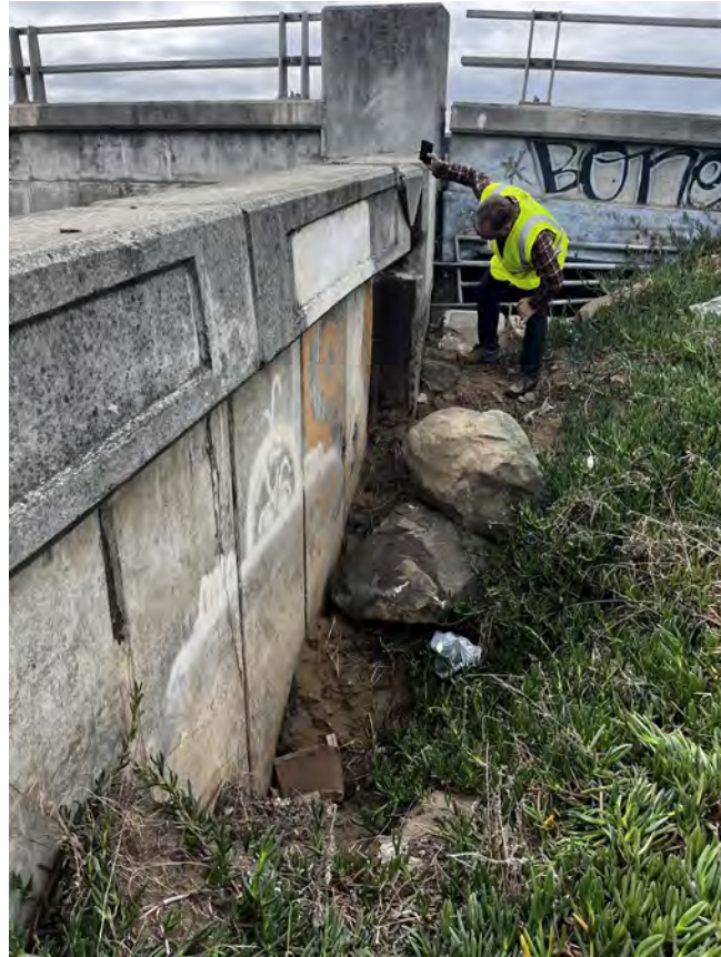
South Creek Bank
