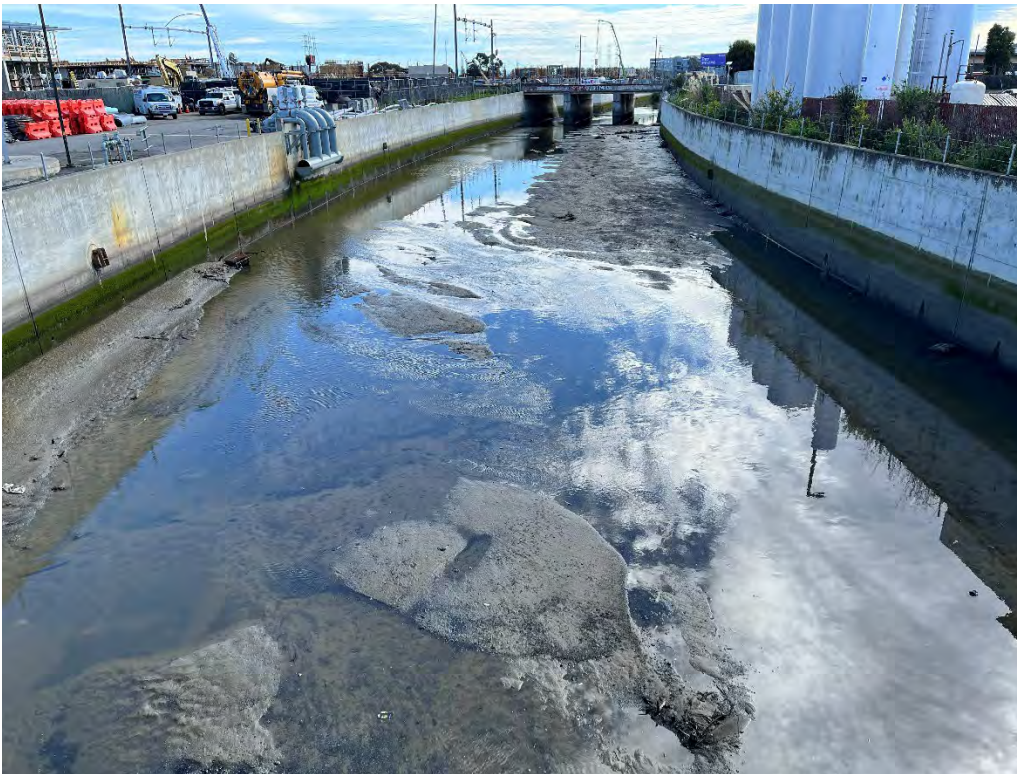
Photos 19 & 20 — Top photo shows Colma Creek looking upstream from Linden Avenue Bridge. Bottom photo shows Colma Creek looking downstream from the Linden Avenue Bridge. Low Tide.
