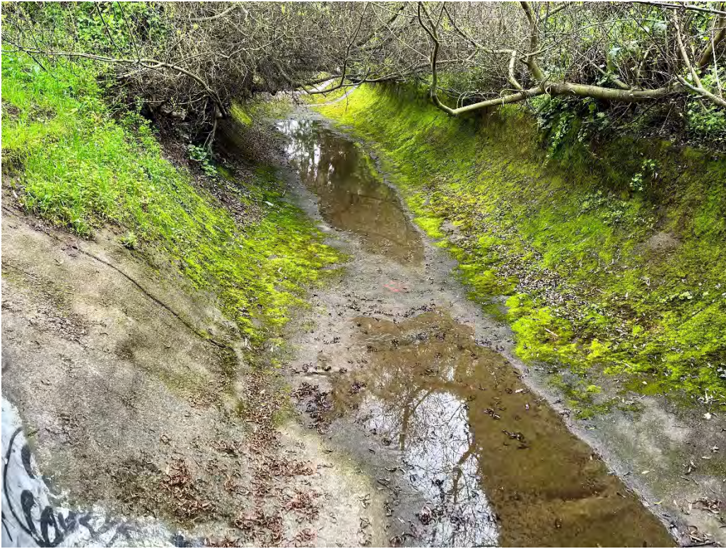
Photos 36 & 37 — Top photo shows Old Colma Creek channel downstream of the El Camino Real Bridge at the Mission Road intersection. Bottom photo shows Old Channel looking downstream from Colma Creek channel.
