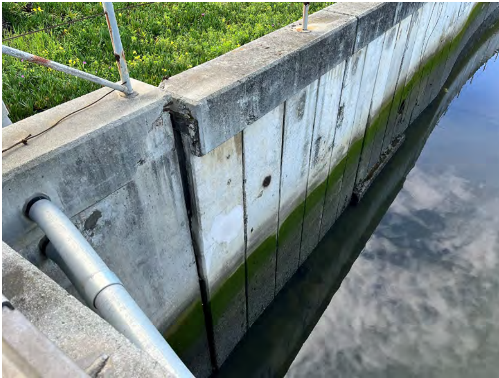
Photos 15 & 16 — Top photo shows void outside channel wall downstream from the Produce Avenue bridge facing the Highway 101 crossing, and bottom photo shows damage to channel wall upstream of Produce Avenue Bridge.
