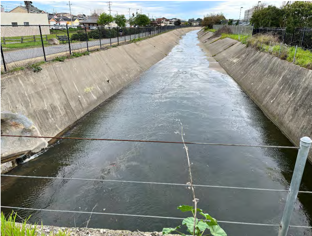
Photos 30 & 31 — Top photo shows damage to channel fence downstream from the BART culvert. Bottom photo shows Colma Creek looking downstream from the BART culvert.
