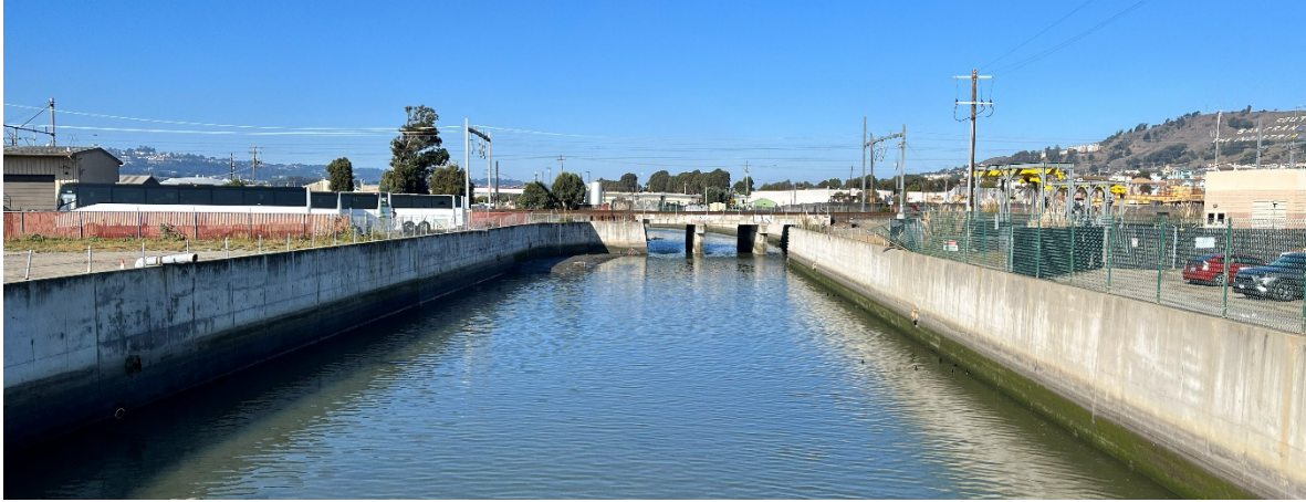
Upstream of San Mateo Avenue, typical reach for sediment removal from above channel
