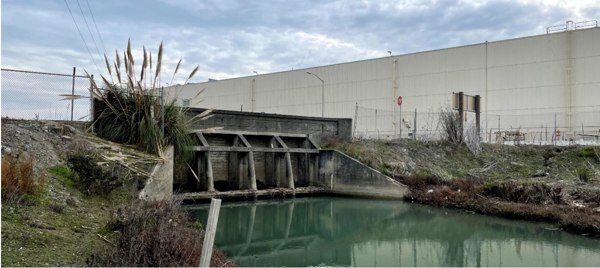
San Bruno Creek Tide Gate at North Access Road
