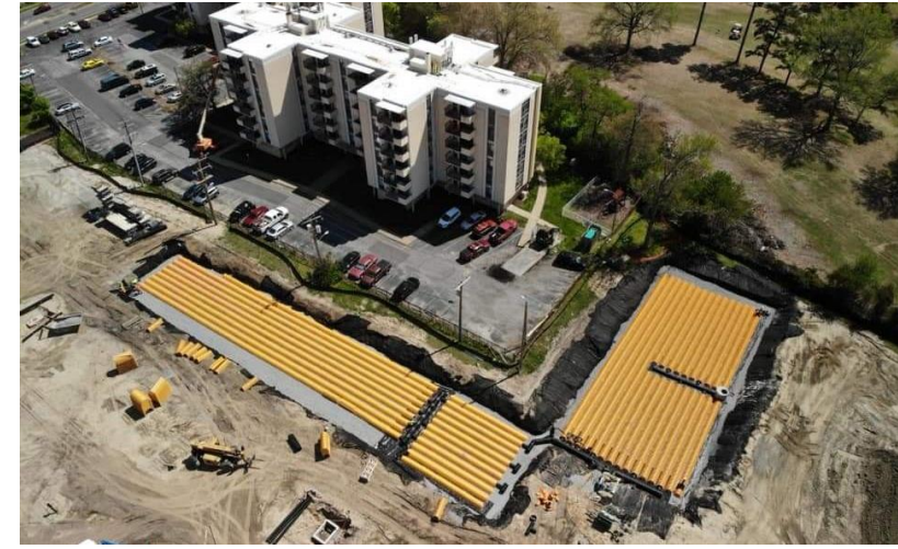
Subsurface detention systems under new development
