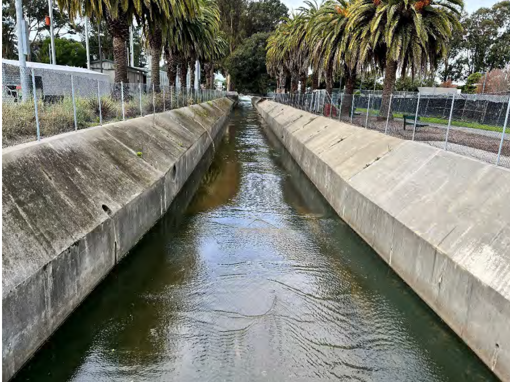
Photos 22 & 23 — Top photo shows the dissipater teeth. Bottom photo shows Colma Creek looking upstream from Orange Avenue Bridge
