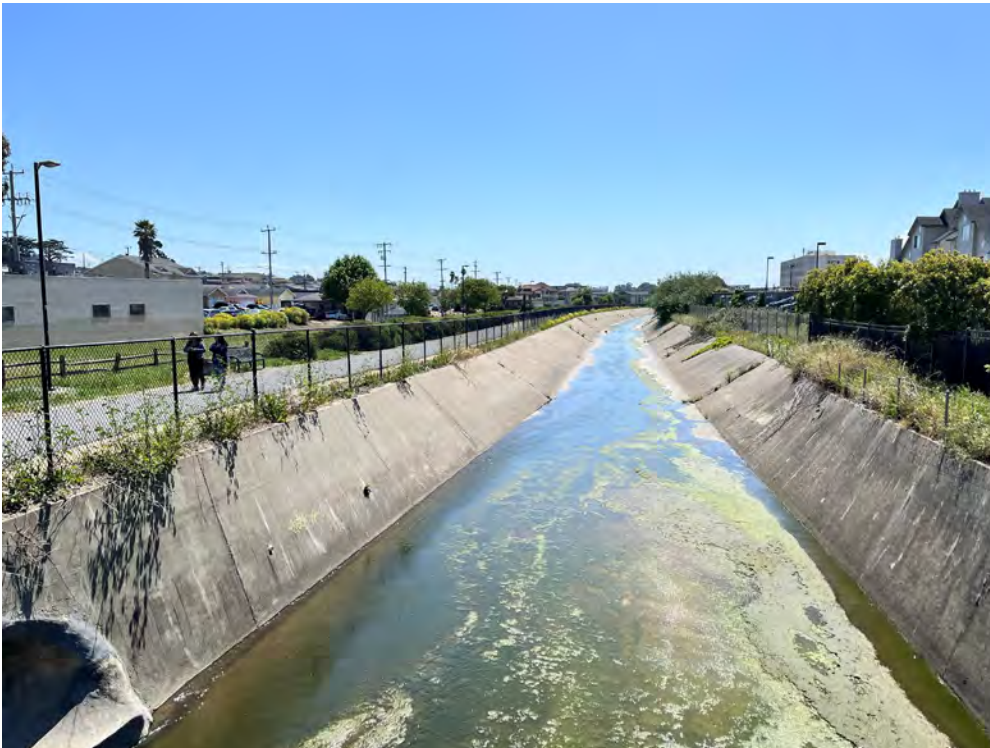
Photos 30 & 31 — Top photo shows vegetation growth over outfalls downstream from the BART culvert. Bottom photo shows Colma Creek looking downstream from the BART culvert.
