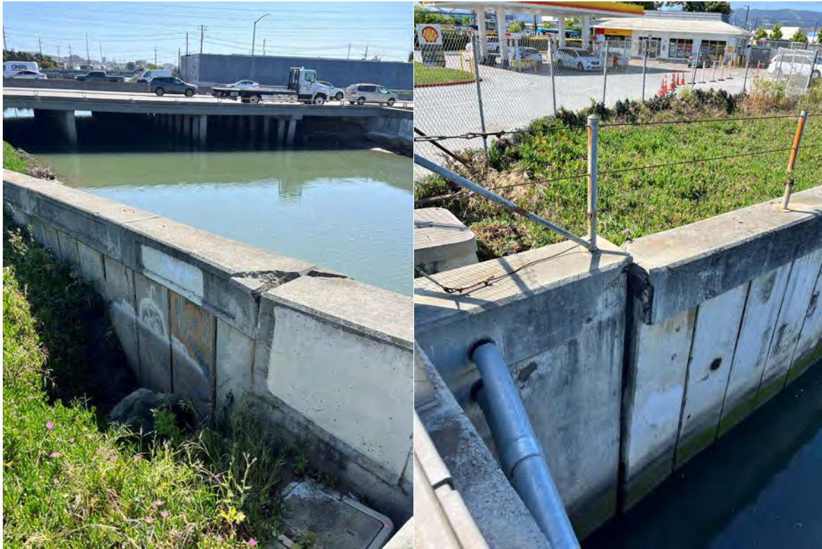
Photos 15 & 16 — Left photo shows void outside channel wall downstream from the Produce Avenue bridge facing the Highway 101 crossing, and right photo shows damage to channel wall upstream of Produce Avenue Bridge.
